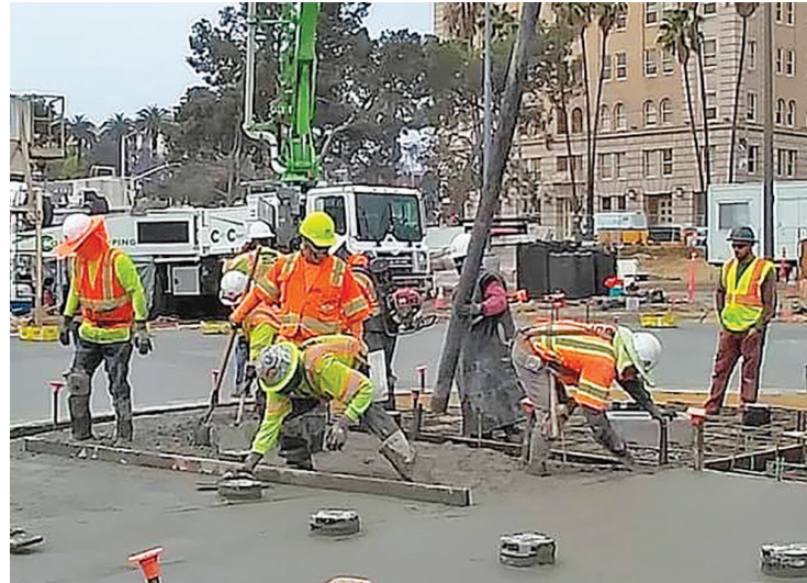
Local 600 members on the job. See back page for more photos from around Southern California.
